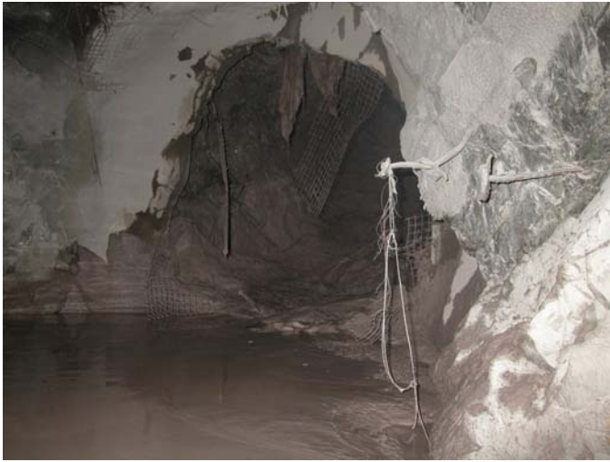
Fig. 4. Photograph of bulkhead failure 1.
