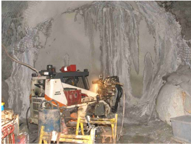
Fig. 1. Fibrecrete bulkhead. Bobcat drill rig shown coring paste from behind the bulkhead.
