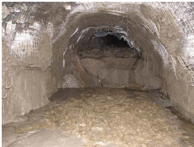
Fig. 15. Failure 2 incident scene.
