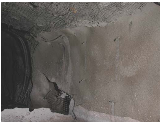
Fig. 7. Photograph of bulkhead Failure 3.
